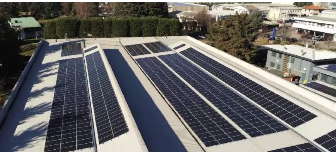
Photovoltaic system at the Saronno plant. Power: 400 kWh
